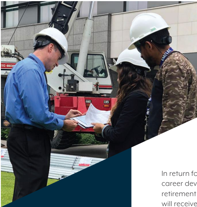
Facility Manager reviewing the contractor's lifting plan to make sure it met EM-385-1-1 requirements at U.S. Embassy Quito.
