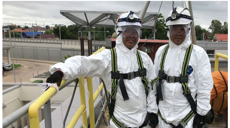
U.S. Embassy, Vientiane Lao PDR: Facilities Maintenance Plumbers wear full body protection for working inside water tank.
